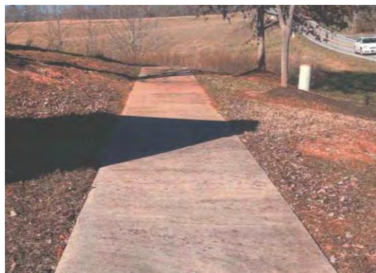
CVS sidewalk that ends abruptly
