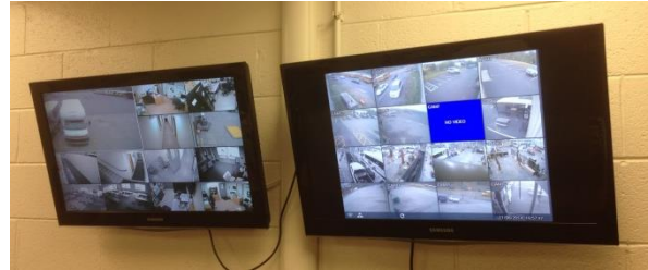
Surveillance at Danville Transit Operations Facility
